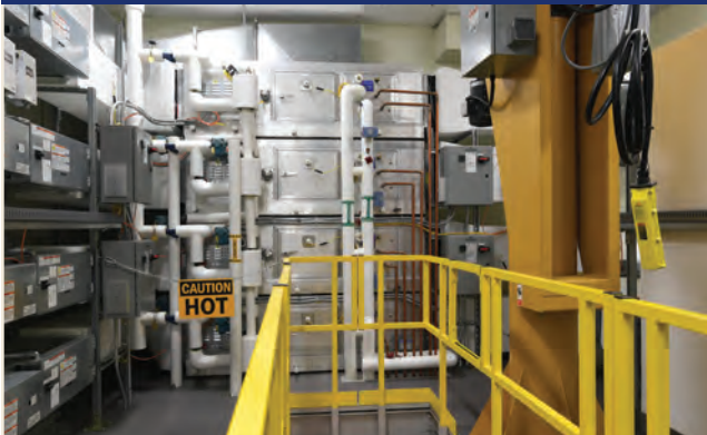
The IBAL contains four simulated zones, stacked one above the other at the center of this image, that generate cooling loads for the water system. Each zone is connected to a VAV unit, shown at the left.
