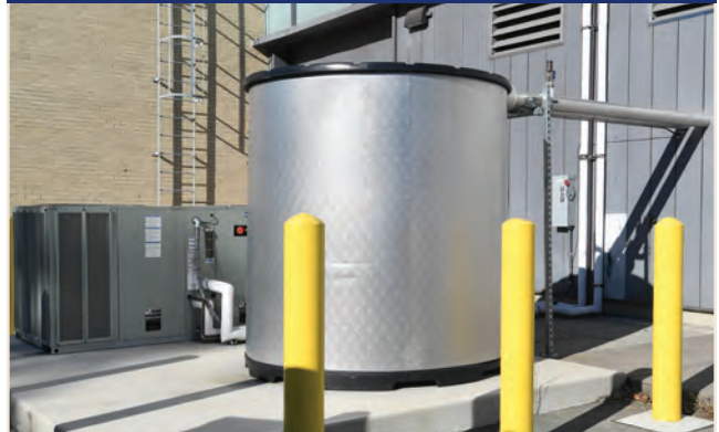
An ice storage tank can be used to meet the cooling loads instead of the chillers or water side economizer. This system allows loads to be shifted to times of the day when electric rates are lower.
