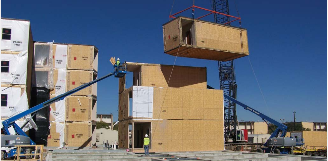
Modules are picked from a carrier bed by a crawler crane and stacked on top of each other with no additional structure. Crews install eight to 12 per day.
