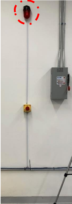
North wall EMO and shutter open indicator light
