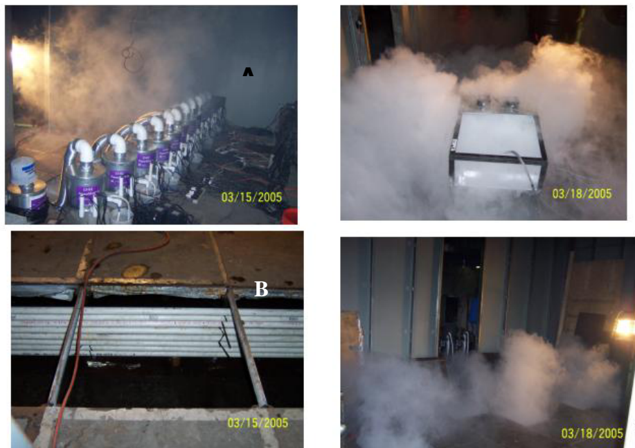
Figure 1: A) UFM-NanoMist® operation in 25 m 2 sub floor, B) tube bundles as obstructions additional to the main baffle, C) electronic cabinet exposed to NanoMist®, and D) NanoMist® leaking out of missing floor tiles.
