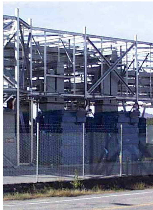
Typical H.V. Transformers
