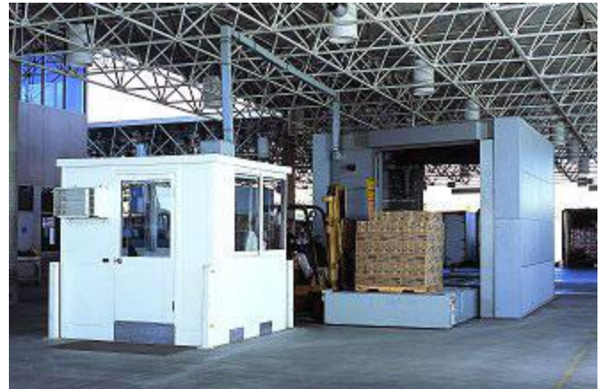
Figure 2R. Cargo screening equipment installed at an airport facility.
