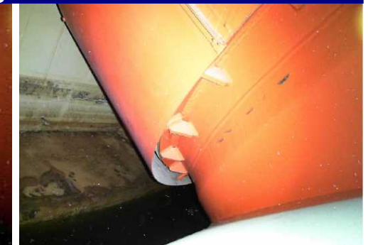
Bottom of venting pipe bellows cover
