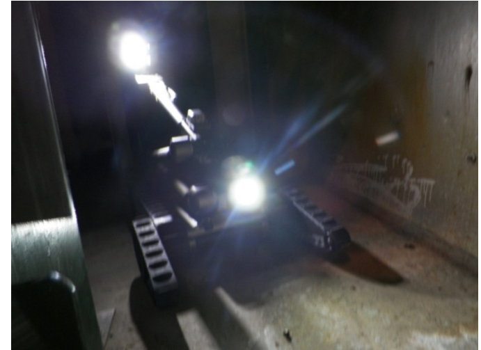
H. B. Robinson's 510 PackBot ® , "Jake" conducts visual inspections in the Regen heat exchanger
