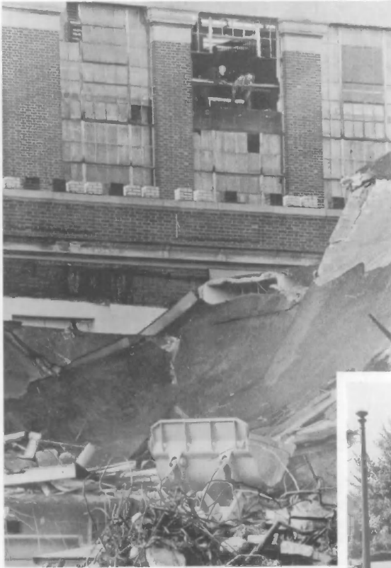
Left: Demolition of the Industrial Building at the old NBS campus. (copyright Washington Post; reprinted by permission of D.C. Public Library)
