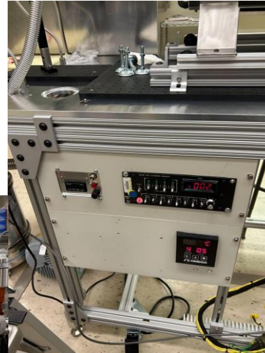
Picture of the controls for the furnace
