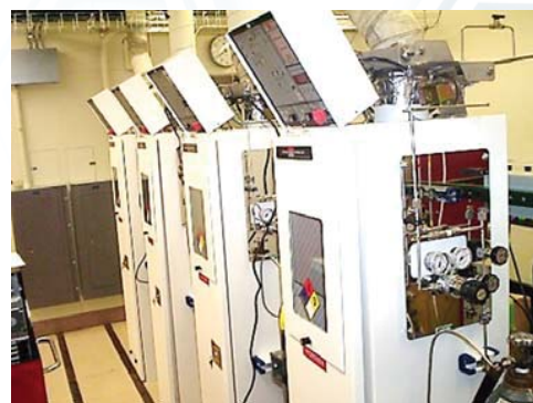
Figure 2. Continuously vented cabinets for hydrogen and methane gas cylinders
