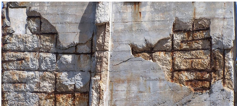
An abandoned building on Northern California's McAbee Beach shows the destructive power of corrosion on a steel-reinforced concrete structure. A new NIST evaluation method using terahertz waves can detect the early stages of corrosion on steel rebars directly through their concrete covering. Credit: Per Loll
