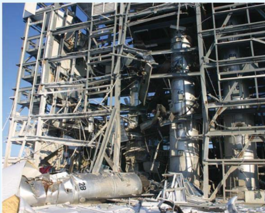
NDK Crystal damage after the incident. The force of the explosion blew out most of the wall panels.
