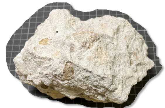
Sample of concrete reported to be “crumbly” by personnel working at collapse site.
