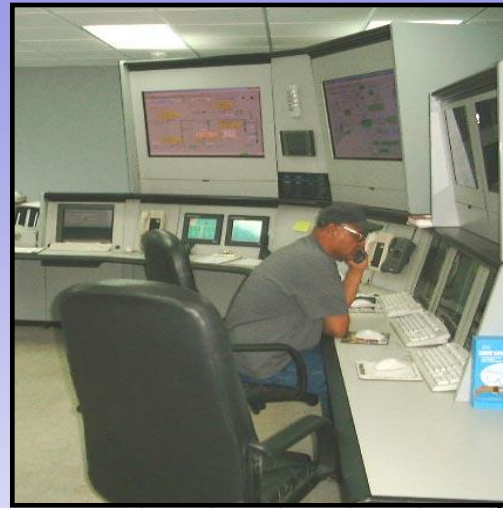
Central Control Room
